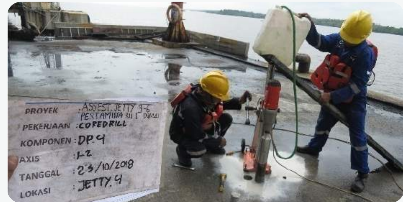
Structural Assessment of Jetty New Plant and Recommendation Development Regarding the Trestle Failure at Jetty New Plant RU II Dumai
